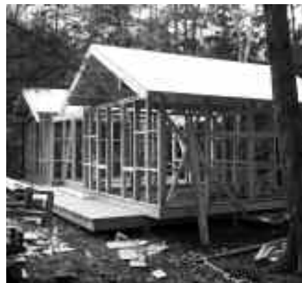
Frame and sheathing of a new cabin are sawed from property trees using a portable band saw mill.
